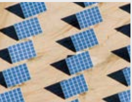
Solar park with 21,000 m 2 of solar module surface, Spain
