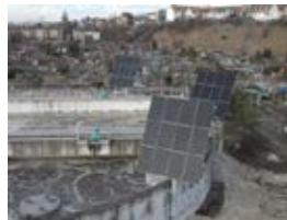
DEGERtracker 3000HD sewage treatment plant Birsfelden, Switzerland
